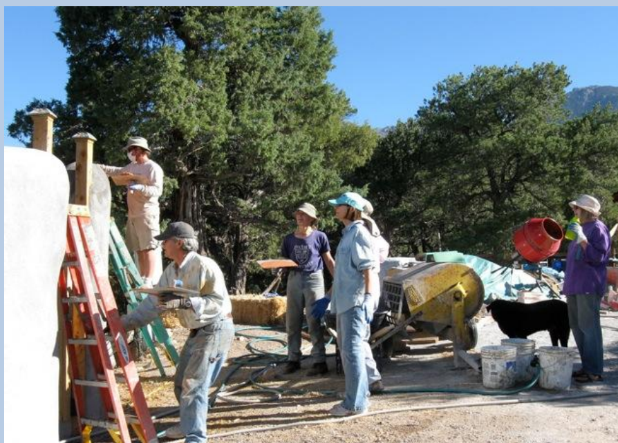
The work party applying the final coat of stucco to the the Great Wall of Crestone
